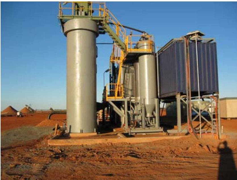
Carbon Tanks, Elution Column and Gold Room
