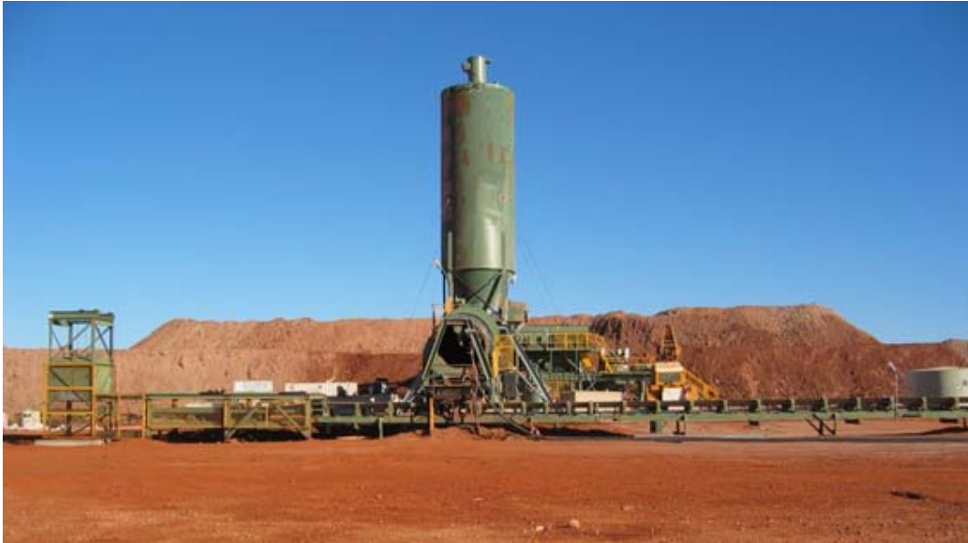
Agglomerator and Cement Silo
